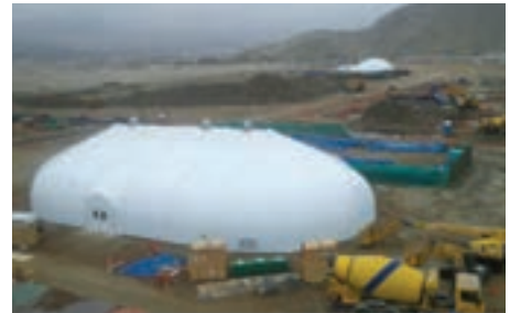
These pre-engineered building systems, initially used as a turbine assembly warehouse (top photo) and a dining facility area (bottom photo), are now integral to plant operations.
