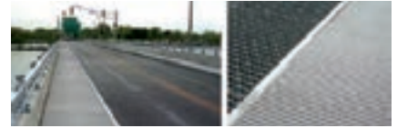
Aluminum extruded plank grating on Grosse Ile Bridge with slip-resistant coating
