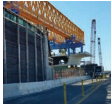
A Reinforced Earth® wall with 5-ft x 10-ft precast panel facing and smooth steel form finish will support the new roadway.
