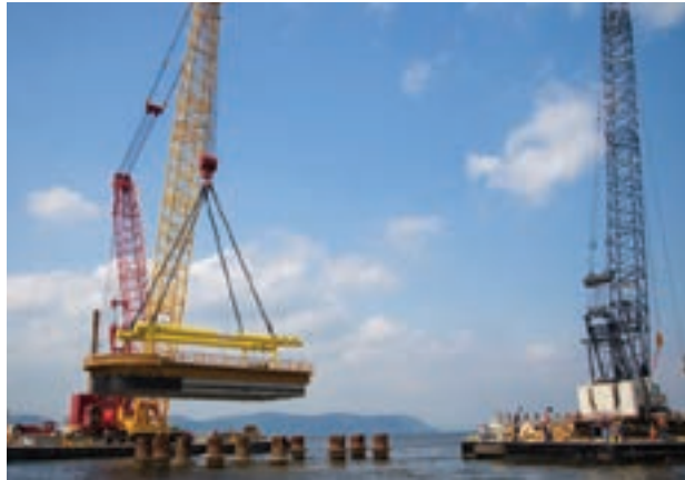
The Hank Hummel 4600 ringer crane sets a precast tub to efficiently form the waterline footings on the New NY Bridge project in Tarrytown, N.Y.
