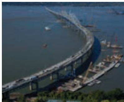
Aerial view of the New NY Bridge project site from Westchester County
