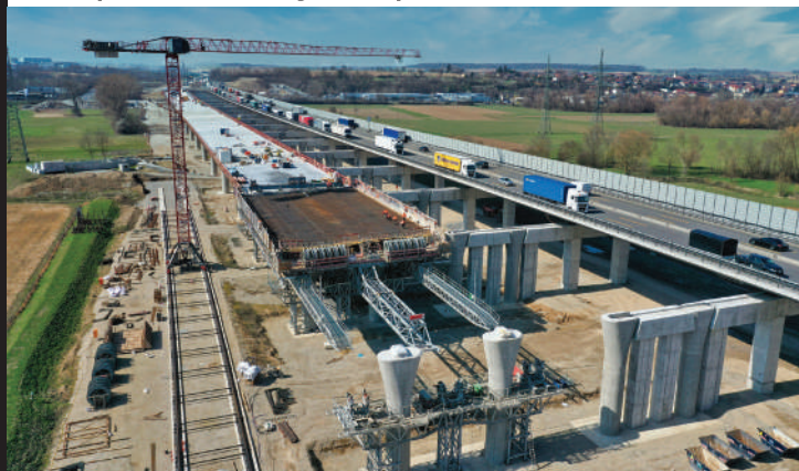
As part of the VIA6West consortium, Hochtief (No. 2) is contractor for the six-lane expansion of federal highway A6 in southern Germany, which will include 36 bridges and noise barriers along the route.
